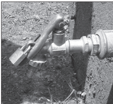
Figure 9.102. The tap can be padlocked.
