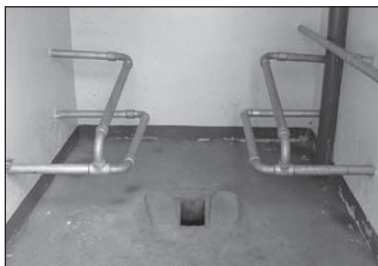
Figure 9.125. Squat latrine with handrails for support.
