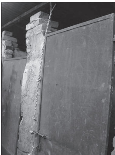
Figure 9.40. Rope hanging from roof beam.
