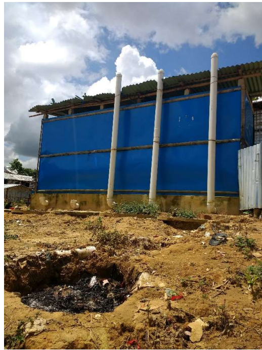
Open waste pit (which is periodically burnt) behind a block of latrines and bathing facilities in Camp 19.
