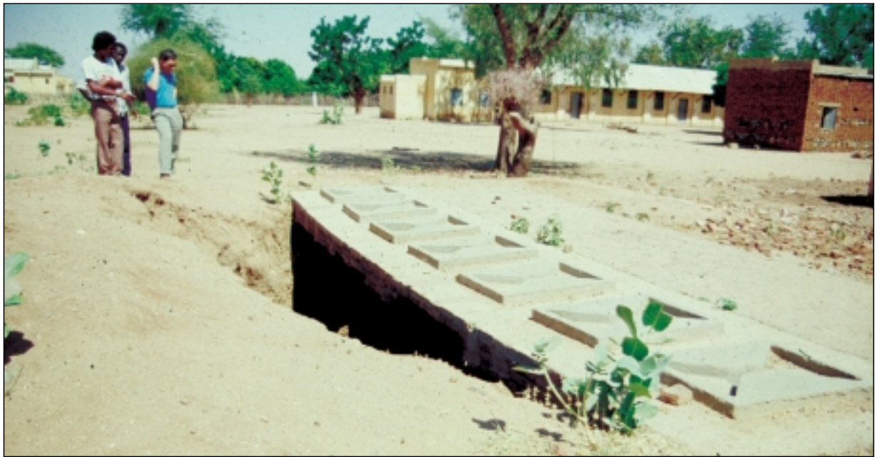
Failed unlined trench latrines, Sudan
