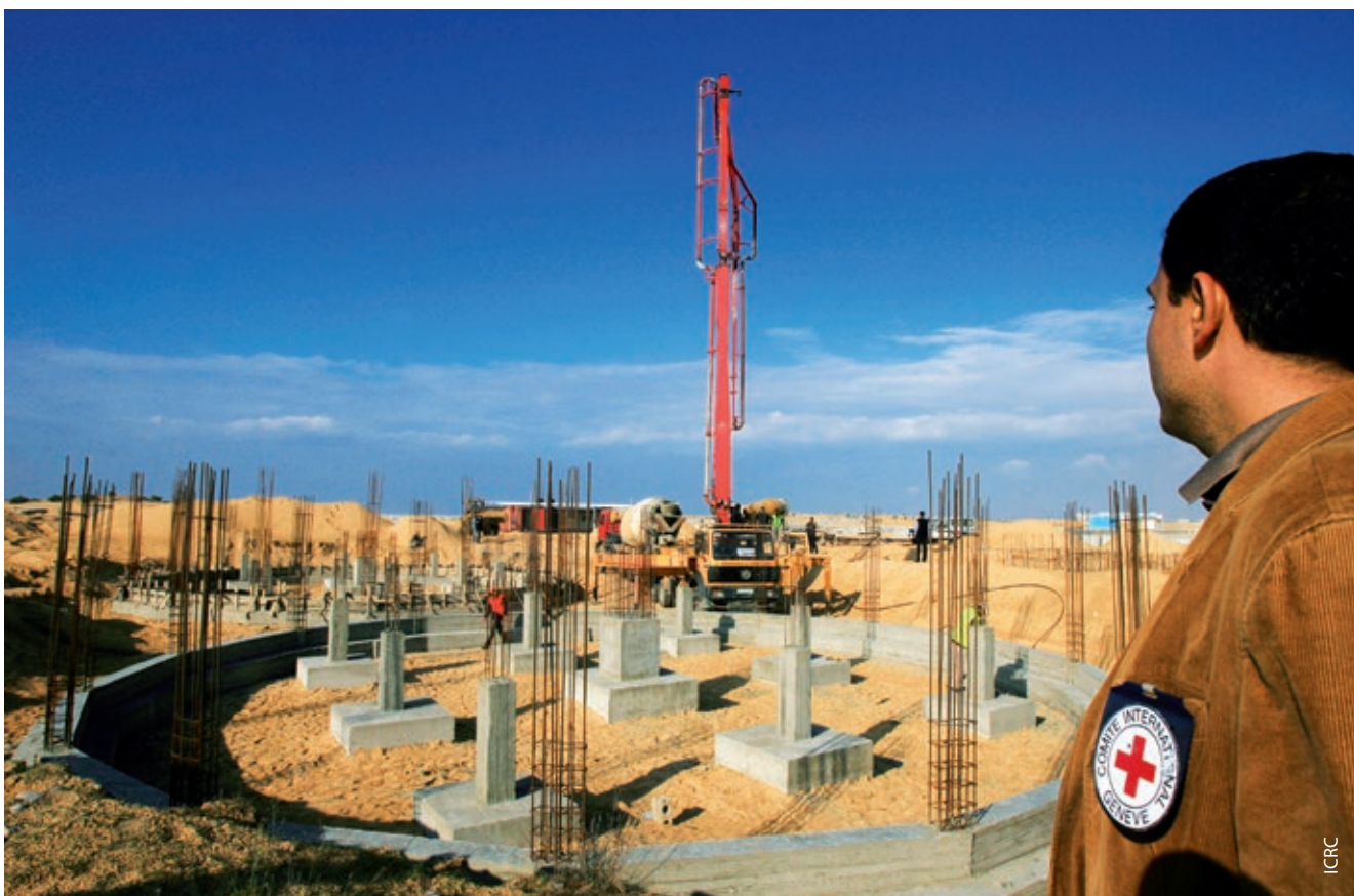
Photo 9. Supervision of the construction by a local contractor of a wastewater treatment plant for the city of Rafah, from which 150,000 residents benefited. (Gaza Strip, 2009)
