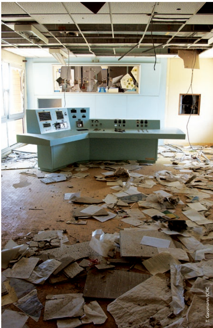
Photo 2. A looted and deserted operation room in a water treatment plant, jeopardizing water delivery for tens of thousands of residents. (Baghdad 2003)
