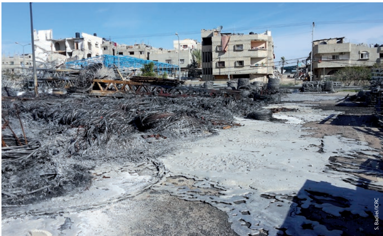
Photo 5. Melted wires and poles resulting from the destruction in 2014 of the warehouse of the electrical company of Gaza, which lost its capacity to react to breakdowns. Necessary repairs to the electricity grid had to be carried out by dismantling items such as transformers, wires and poles at less critical places and placing them in more critical places (e.g. hospitals). (Gaza, 2014)
