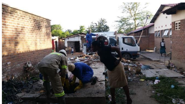
Septic tanks contained a lot of heavy materials and thick sludge.
