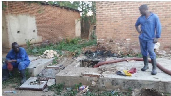
Emptying of septic tanks was a night mare
