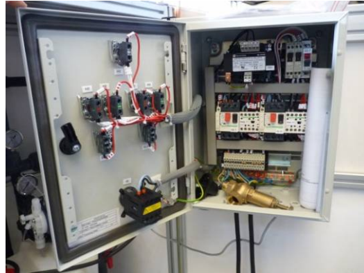
Electrical control Panel. It contains at reception the manuals for the liquid feed pump, the circuit diagram of the control panel, the upper deflecting valves of the filters, and the handle of the control panel door.
