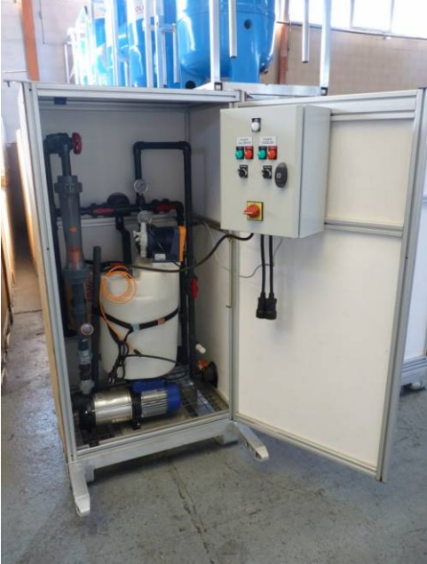
Control panel of the filter, at reception
